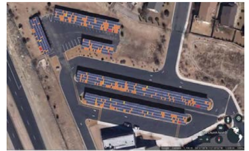
Drone footage of Granville Elementary School solar panel system. All colored panels show areas where the system was not working properly.
